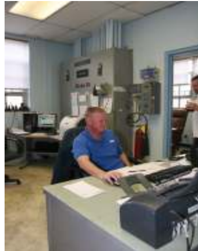
Morgan O'Dell, Senior Wastewater Operator, checking wastewater process status
