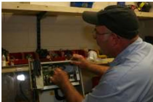
Harry Pool, Utilities Maintenance Mechanic, performing preventive maintenance on an automated chlorine analyzer
