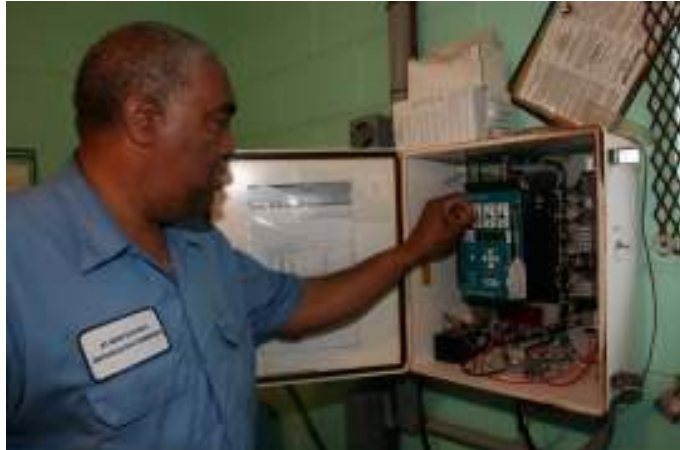
Bobby Moore, Licensed Operator checking controls on a SCADA TCU Unit
