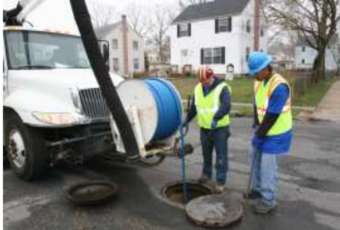
Freddie Swann, VacTor Operator and Thomas Somerville, Maintenance Specialist, performing preventive maintenance on sewer lines
